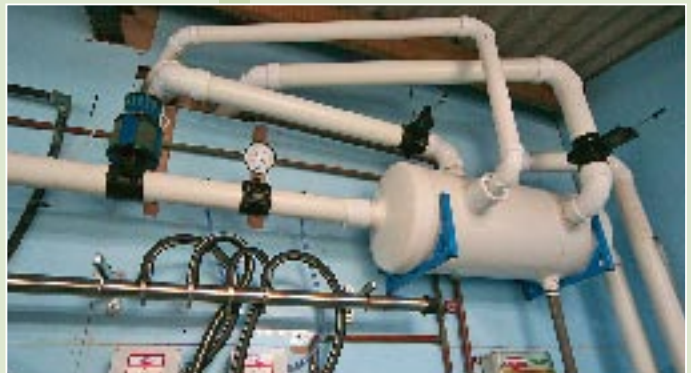
A high-capacity vacuum header tank should be part of any parlour upgrade. This one has a 100-litre capacity and provides separate lines for the parlour’s ACRs, pulsators and clusters, all of which are looped back to the tank.
